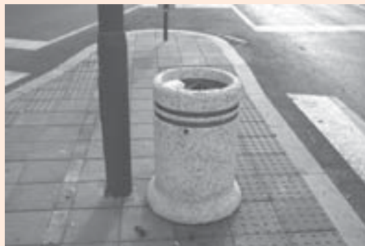
Trash bin obstructs textured pathway
