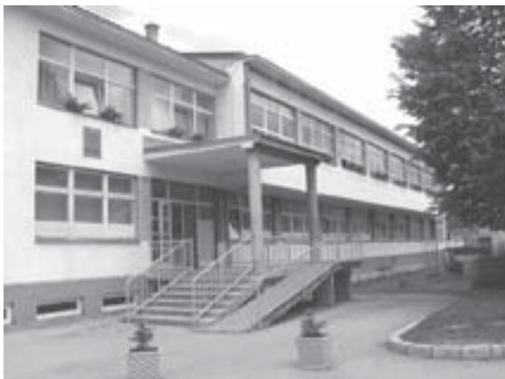
School with ramp but nothing on the interior of the building is accessible, Gorazde, BiH
