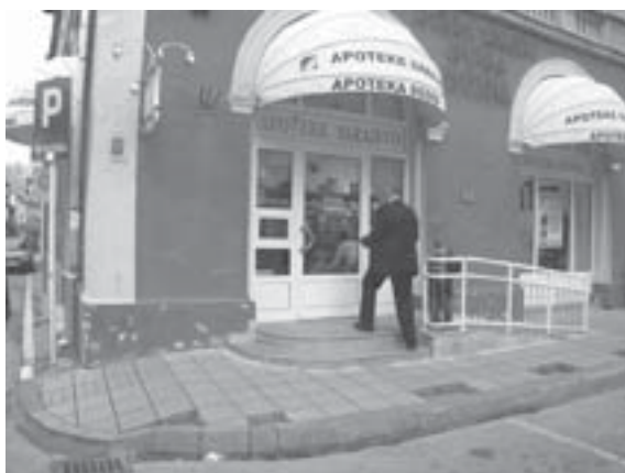
Pharmacy in Sarajevo, the ramp is difficult to use and the kerbs are not cut properly to allow easy access
